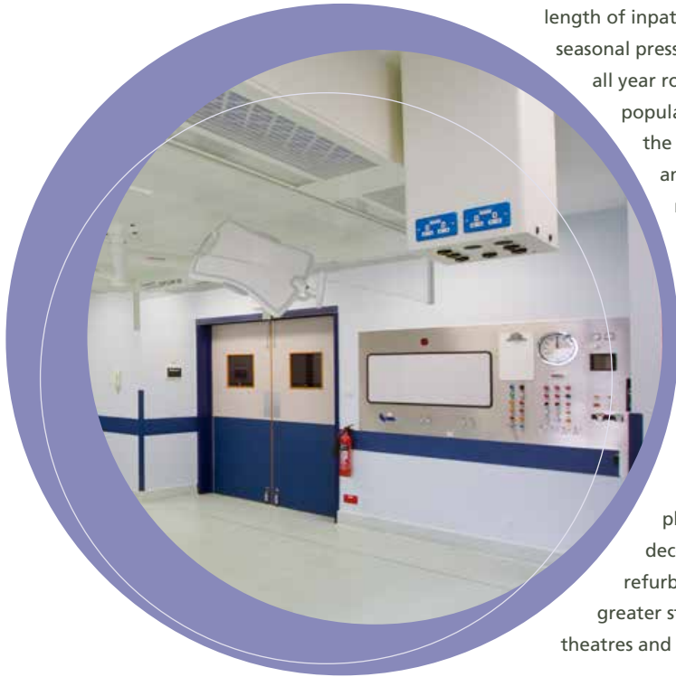
above An interior from one of the refurbished theatres, showing improved layout for greater clinical efficiency
