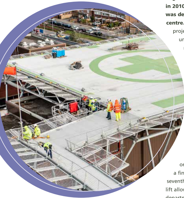
above The helipad at St George's Hospital during the construction phase right Board members and senior management of St George's Hospital with helicopter crew
